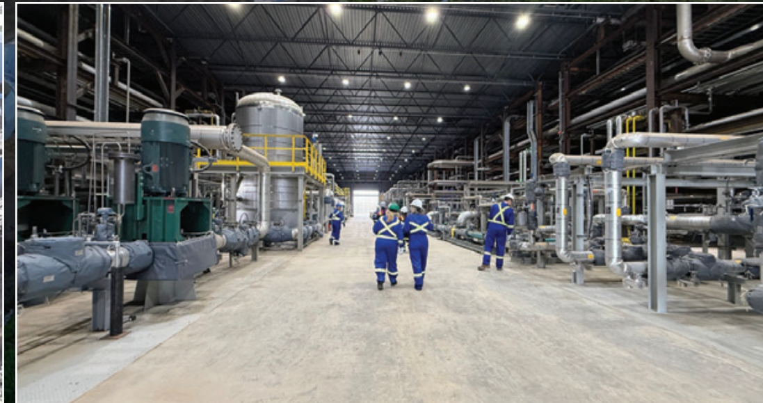
Oil Processing Facilities
